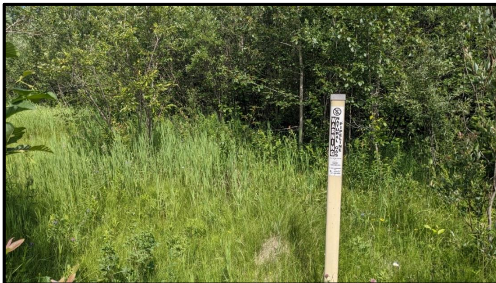
Image 22. Photograph 2892 of a marker indicating the presence of a buried natural gas pipeline along the north side of Oil Tank Road.
